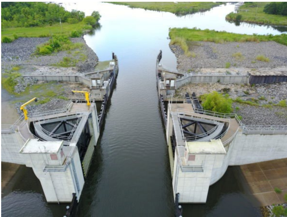
Figure 32: Sector Gate Example (Source: Southeast Louisiana Flood Protection Authority East https://www.floodauthority.org/the-system/bayous-bienvenue-and-dupre-sector-gates/ )
