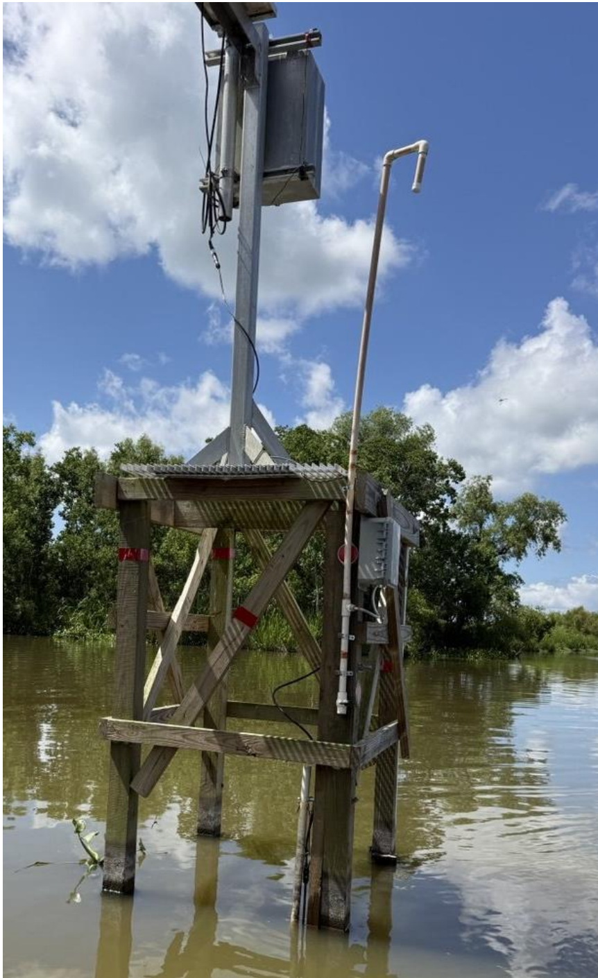
Figure F-3. Photo of CRMS0411-H02 which is mounted onto the USGS four post platform. Survey the CR and SG and be sure to indicate the station is –H02 which differentiates the site from the old USGS real-time station that was on the same platform. Note: No new staff gauge was added when the new station was added to the platform.
