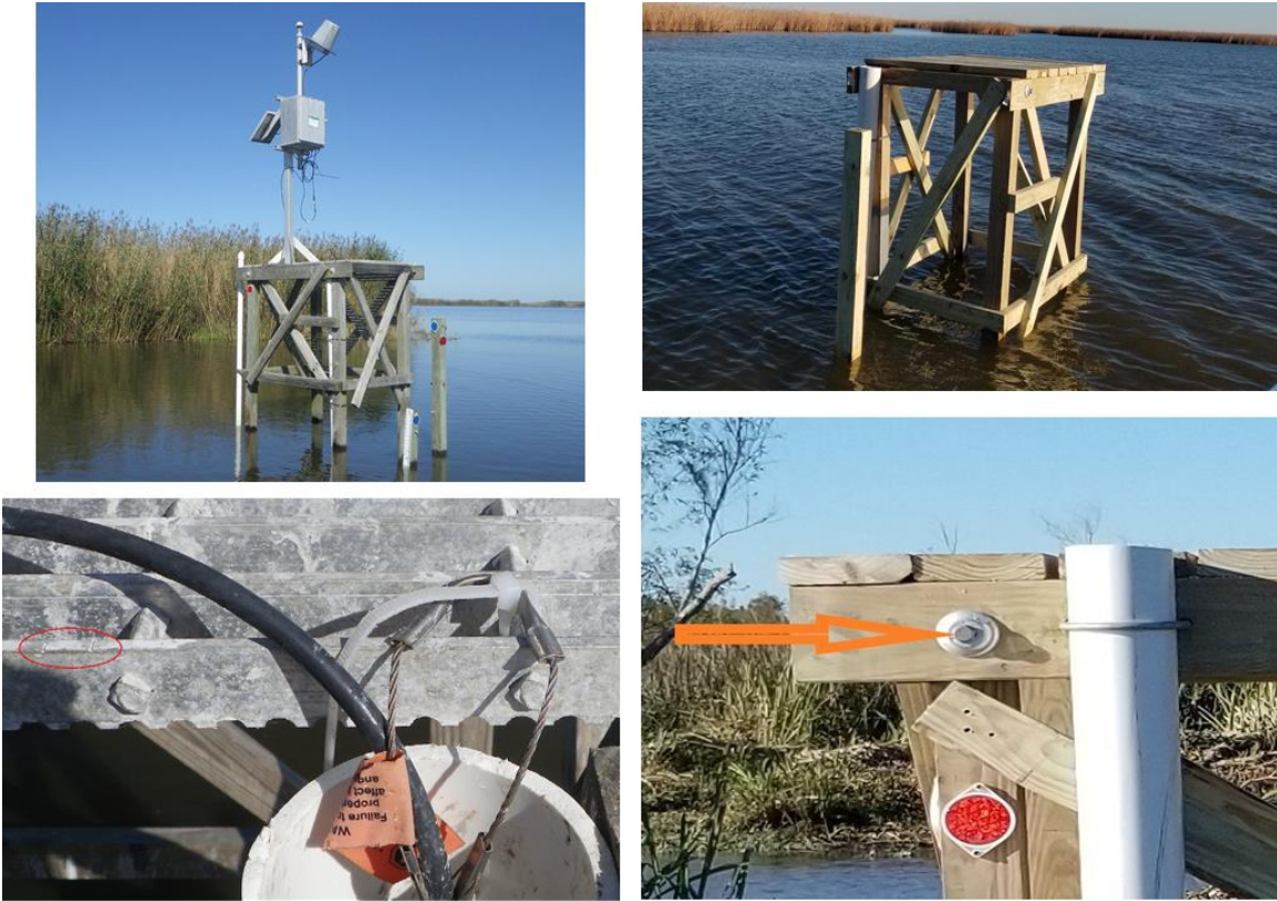
Figure A-7. The photos display USGS/Real-Time (H01-RT) 3' x 5' wooden platforms that function as continuous recorder sites. The continuous recorders are mounted inside the PVC pipes that extend to the top of the platforms. The platforms decks, catwalk grating (left) or wooden (right) have different configurations for the survey “mark”. Note, the detached 4”x4” posts installed next to the platforms (top) are the support poles for staff gauges and the old “typical” sonde post which will also be surveyed.
