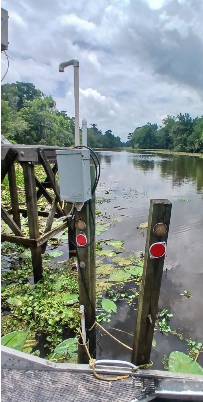
Figure F-1. Photo of CRMS0061-H02 which is mounted on a post next to the old USGS real-time four post platform. Survey the CR and SG as with any other site and ignore the old USGS four post platform.
