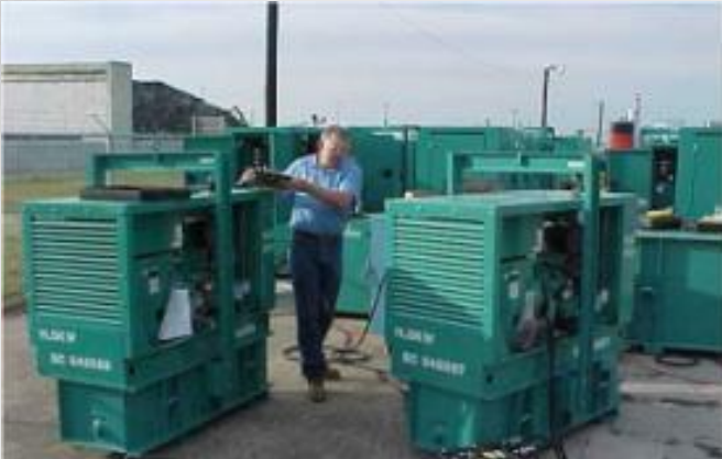
Temp. Emergency Power
