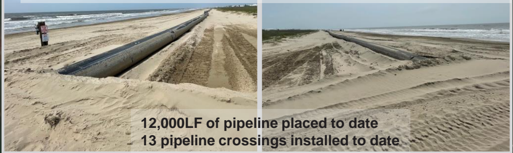
Pedestrian/ATV dredge pipeline crossing
