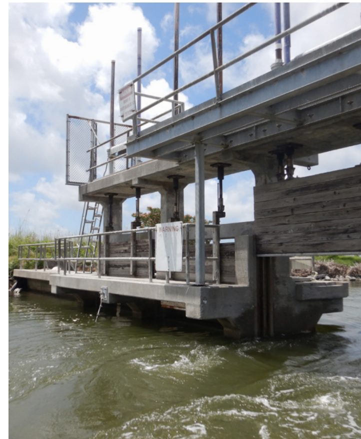
Image: Cameron-Creole Hydrologic Control Structure, 2022 (CPRA)
