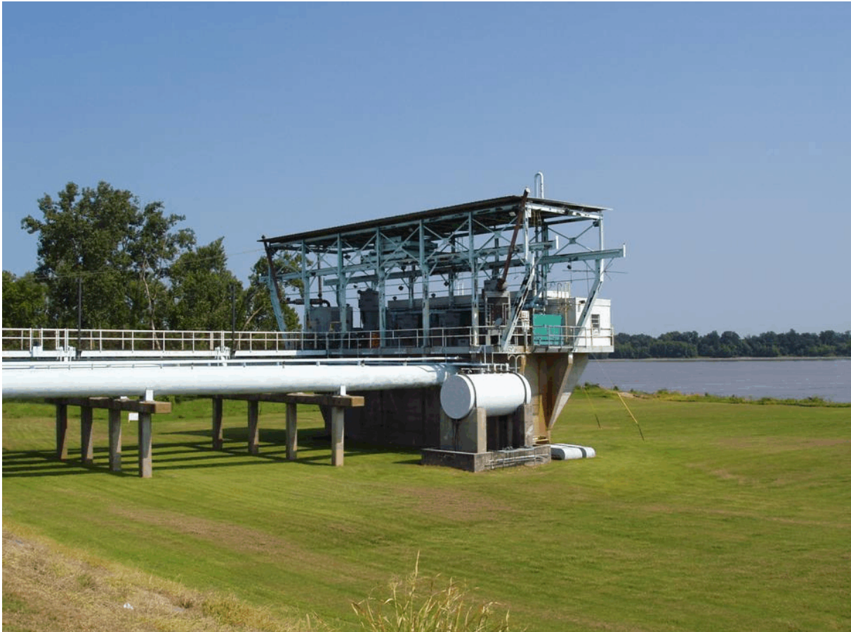
Figure 6.1: Pump Station at Donaldsonville
